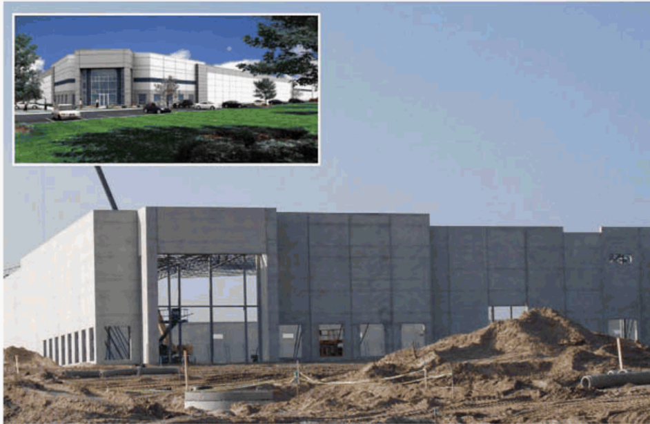
The 574, 249 sf MidPoint USA spec building in AmeriPlex at the Port in Portage is nearing completion and will be ready for build out in the summer of 2008.
